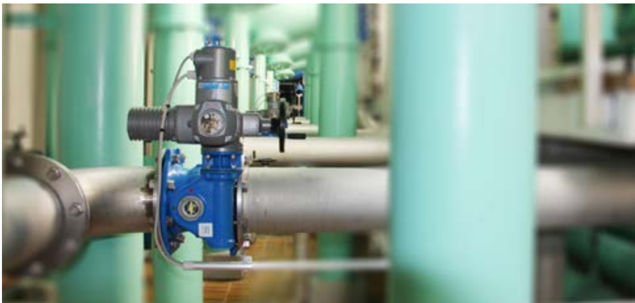
INSTALLATION AT THE DRINKING WATER TREATMENT PLANT IN SINDELINGEN, GERMANY
